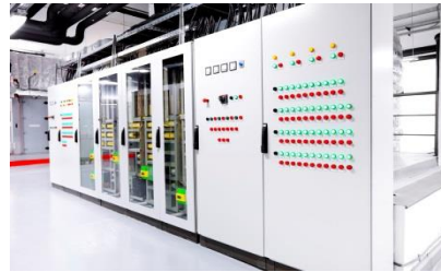
Bldg. Automation & UPS
